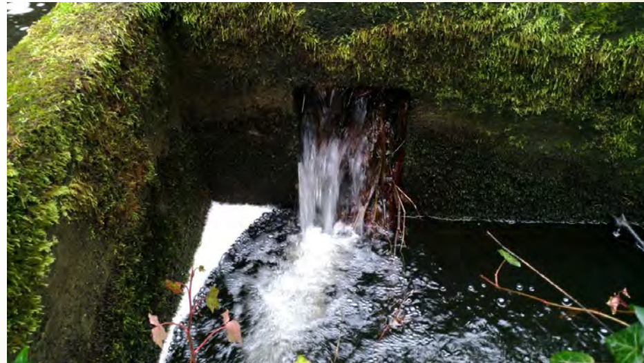
Example of debris that plugs up fish ladders.
