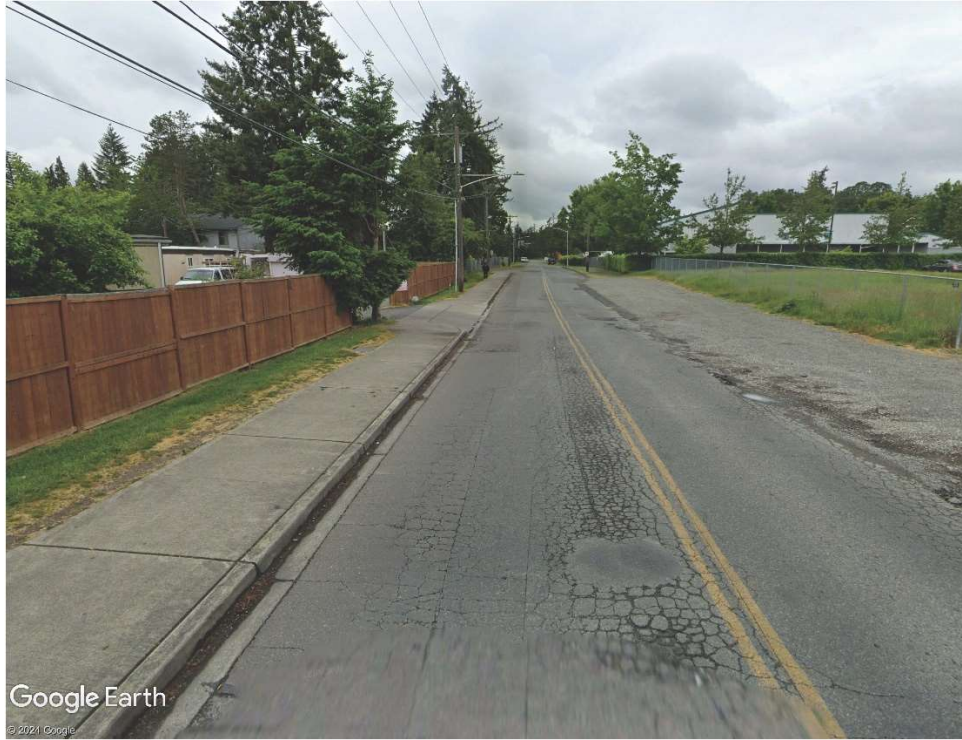
Before – Image Date: August 2018 (Credit: Google)
