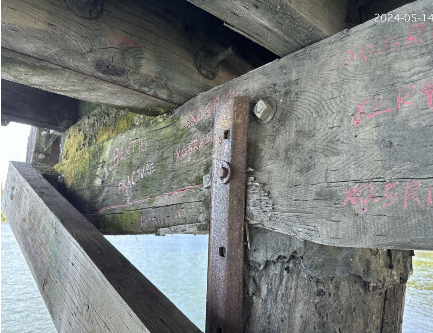
Cap is pulling the deck down in this condition, causing harm to surrounding members
