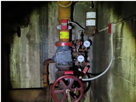
Theater Fire Suppression Manifold
