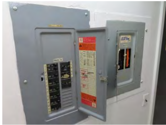
Newer Electrical Service Panels
