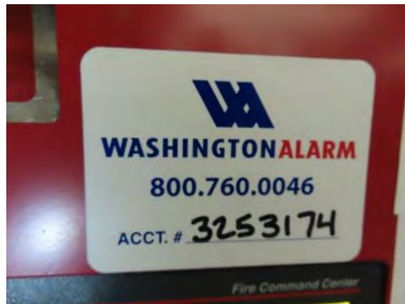
Fire Alarm Control Panel Maintained by Washington Alarm
