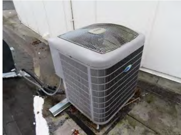
Carrier 5-Ton Heat Pump (No Age Listed, but Old)
