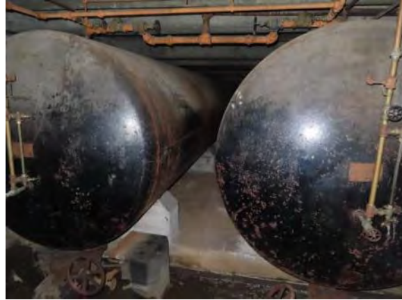
Abandoned Water Tanks for Fire Suppression System
