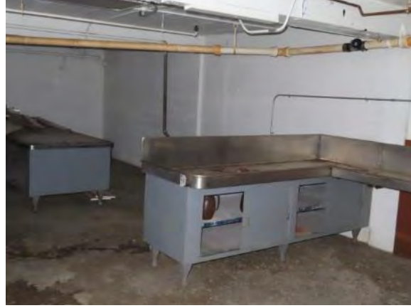
Abandoned Kitchen Equipment
