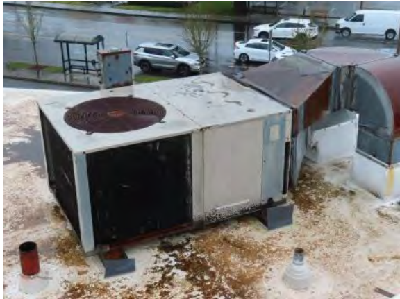
Lennox 7.5-Ton Roof Top HVAC Unit (No Age Listed, but Old)
