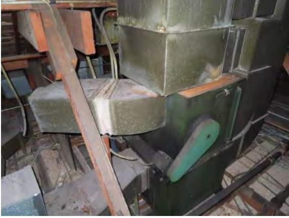
Abandoned HVAC Unit in Theater Attic
