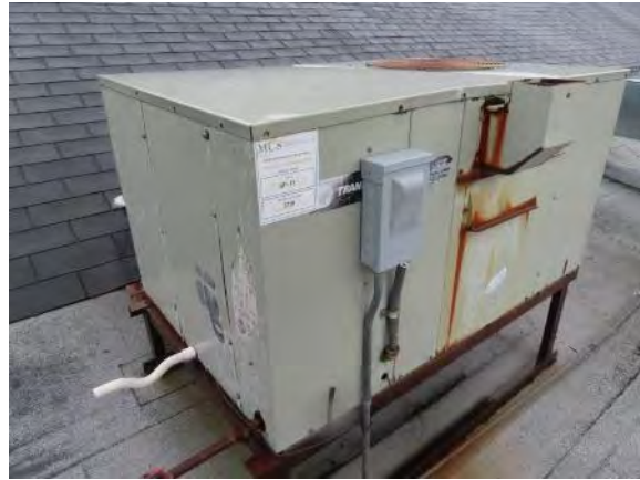
Trane 5-Ton Roof Top Single-Package HVAC Unit, No Age Listed but Old
