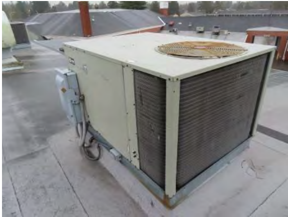
Trane 5-Ton Single-Package HVAC Unit Manufactured in 2000
