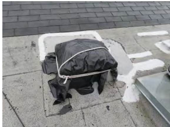
Improperly Capped Roof Opening
