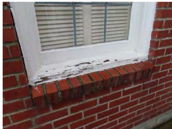
Typical Trim in Need of Paint
