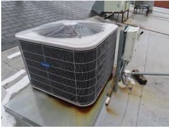
Old Carrier HVAC Unit (Assumed 3-Tons)
