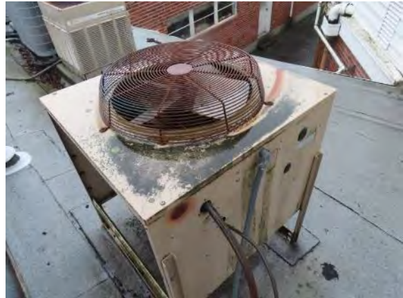
Abandoned Refrigeration Equipment
