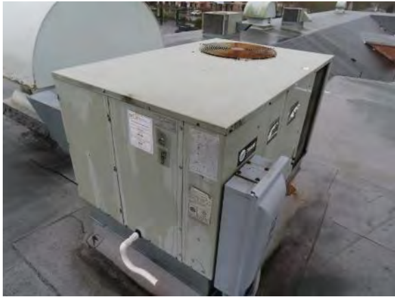
Trane 3-Ton Single-Package HVAC Unit Manufactured in 2000
