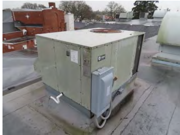
Trane 5-Ton Single-Package HVAC Unit Manufactured in 2000
