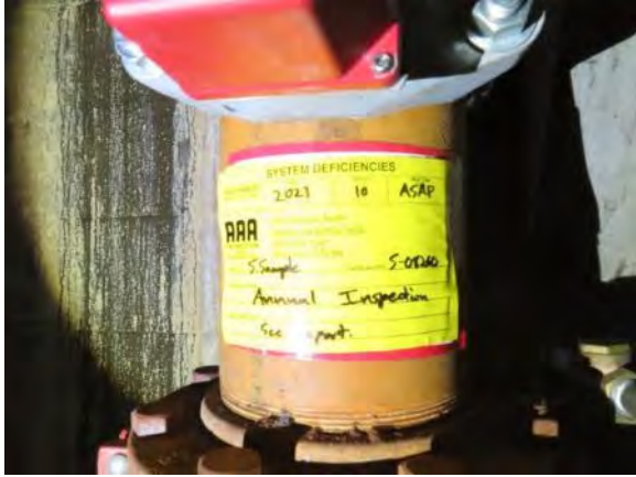
Old Yellow Tag Following Theater Sprinkler Failure
