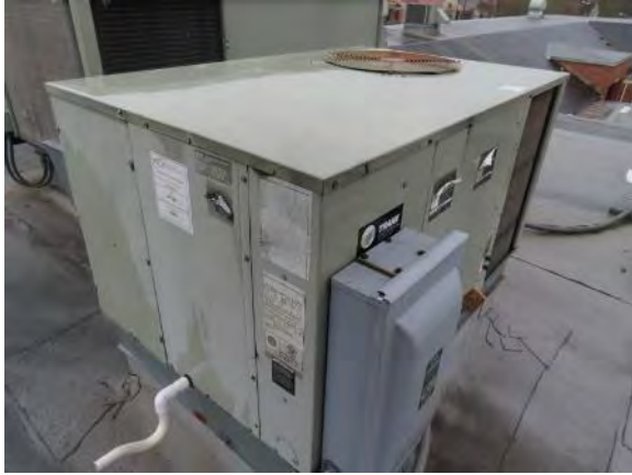
Trane 3.5-Ton Single-Package HVAC Unit Manufactured in 2000
