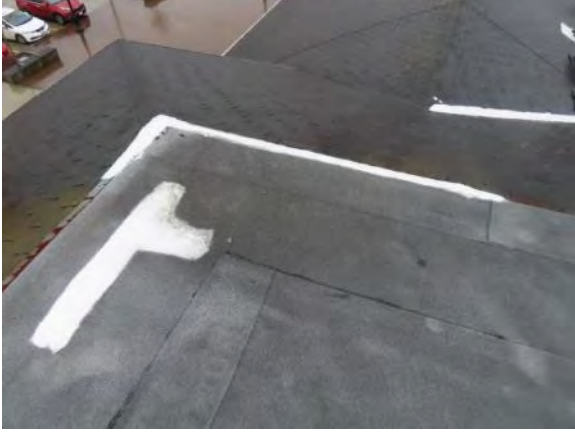
Former Patches on Areas of Leakage
