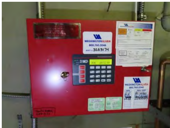
Fire Alarm Control Panel
