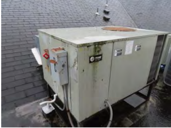
Trane 3-Ton Single-Package HVAC Unit Manufactured in 2000
