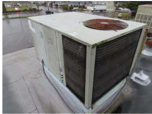
Trane 3-Ton Single-Package HVAC Unit Manufactured in 1998
