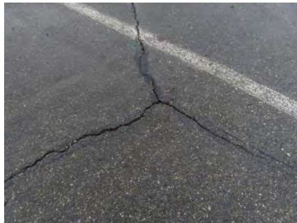
Rubber Crack Sealing Needed in Many Areas
