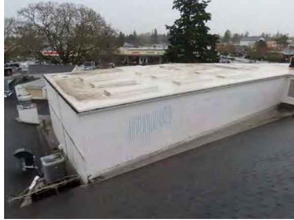
T1-11 Plywood Siding is Poor on Theater
