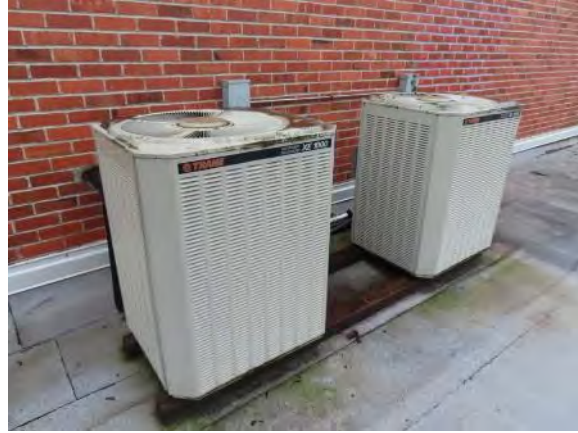
Two Trane 5-Ton Heat Pumps Manufactured in 1992
