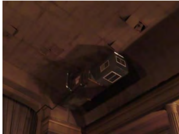
One of Two Air Handlers in Theater
