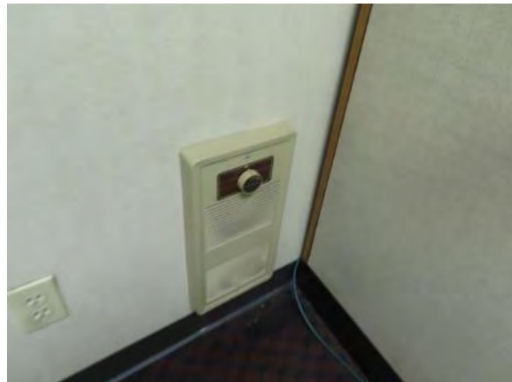
Typical Electric Wall Heater
