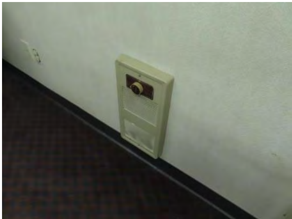
Typical Electric Wall Heater
