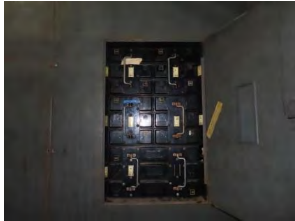
Main Breakers in Theater Basement
