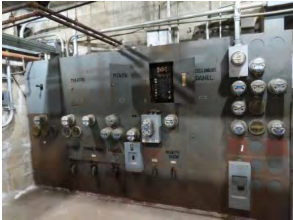
Older Switchgear in Theater Basement
