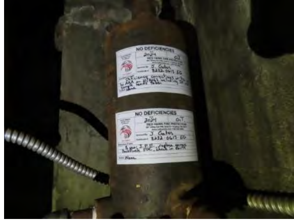
Subsequent Tag on Theater Suppression System with "No Deficiencies" Listed
