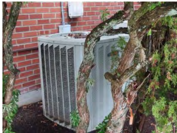
Trane 3.5-Ton Split-System Heat Pump Manufactured in 2008
