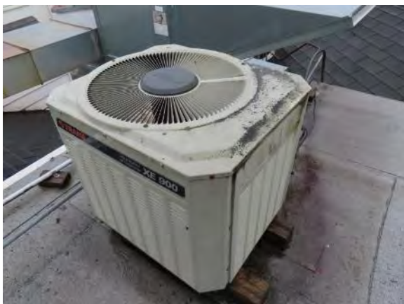
Trane 5-Ton Heat Pump (No Age Listed, but Old)
