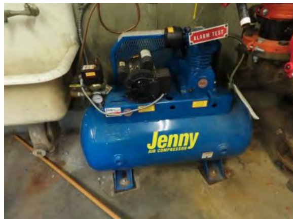
Dry System Compressor Adjacent the Dry System Manifold
