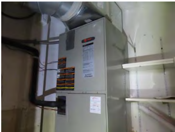
Trane Split-System Heat Pump Air Handler for Unit 9514D
