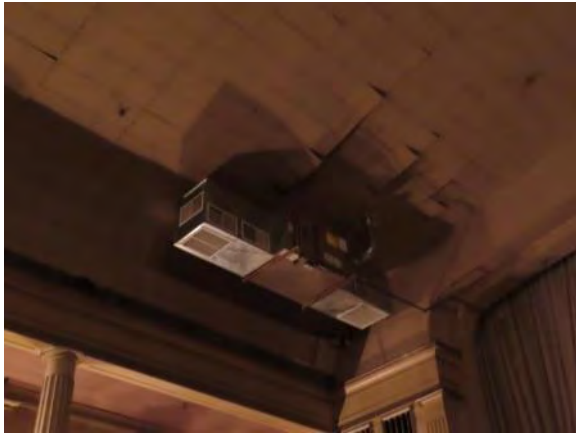
One of Two Air Handlers in Theater
