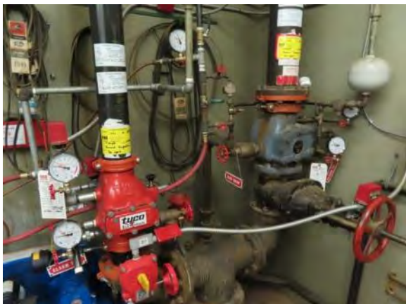
North Fire Suppression Manifold
