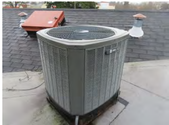
Trane 3-Ton Heat Pump Manufactured in 2014
