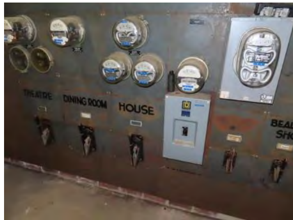
Main Disconnects on Theater Switchgear
