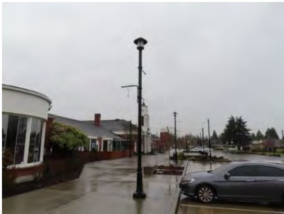
Typical Pole Mounted Street Light
