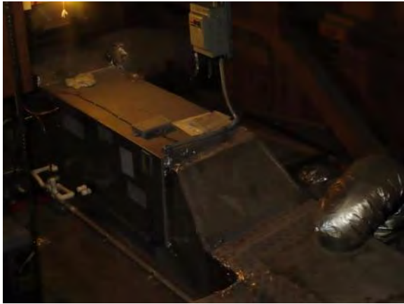
Trane Furnace in Theater Attic
