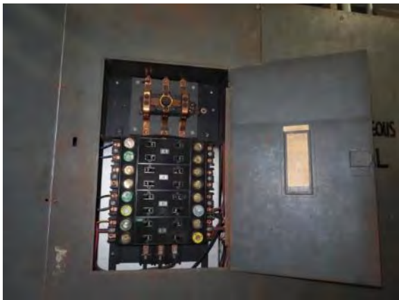
Fuse Boxes in Theater Basement
