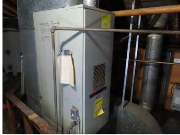
Trane Furnace in Theater Attic
