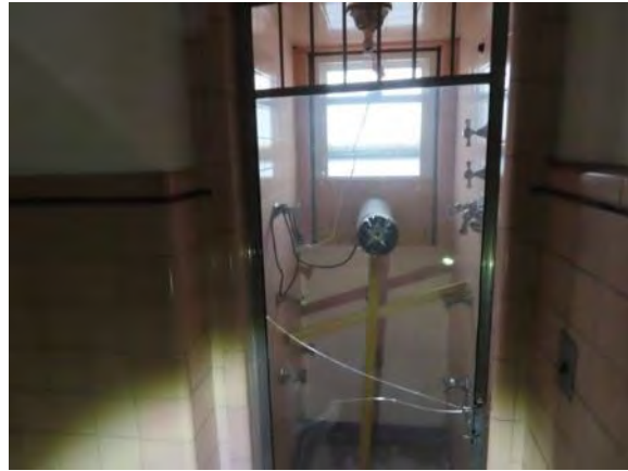
Bizarre Ventilation Apparatus in Dentist Office Shower
