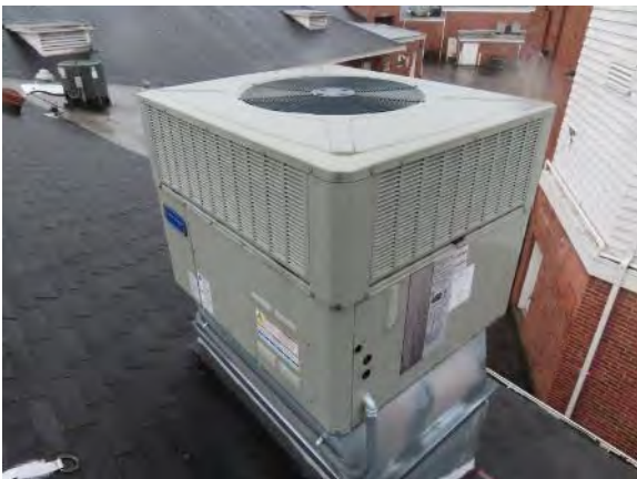
Trane 2.5-Ton Single-Packaged HVAC Unit Manufactured in 2022
