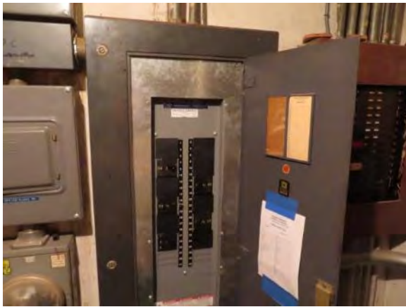
Older Style Electrical Service Panel
