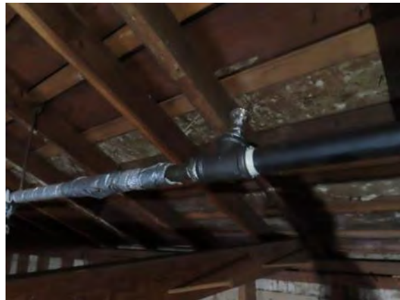
Typical Fire Sprinkler in Theater Attic
