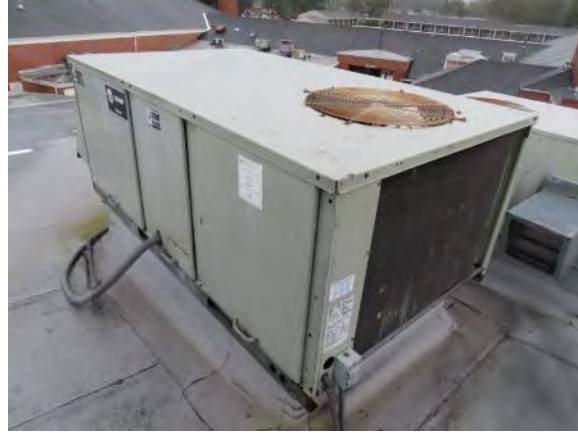
Trane 7.5-Ton Single-Package HVAC Unit Manufactured in 2000
