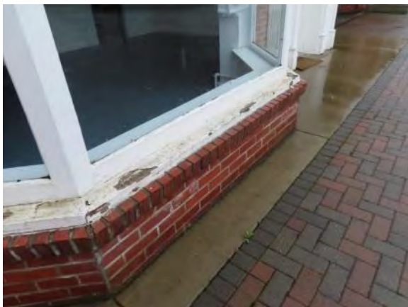
Typical Trim in Need of Paint
