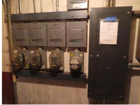
Older Panels and Meters
