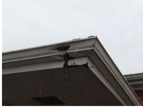
Leaking Gutter at the NE Corner, Typical of Many Areas
