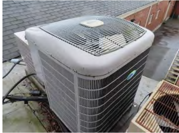
Carrier 5-Ton HVAC Unit (No Age Listed, but Old)
