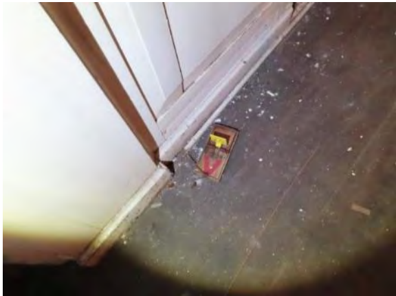
Rodent Traps, Rodents, and Droppings Present Throughout Unoccupied Spaces and in Some Occupied Spaces
