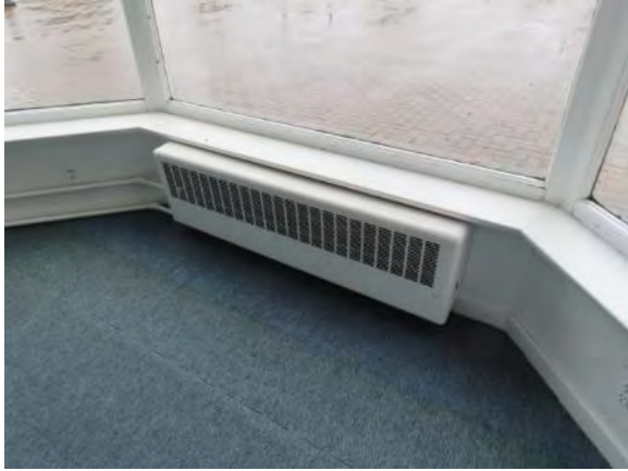
Abandoned Hydronic Heater
