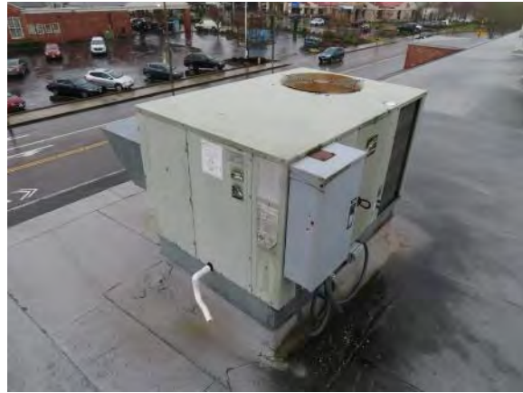
Trane 3-Ton Single-Package HVAC Unit Manufactured in 2000
