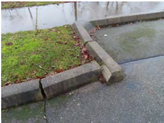
Typical Extruded Concrete Curbing in Need of Repairs
