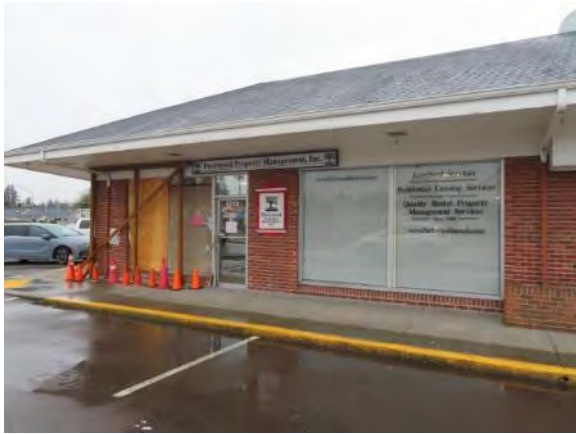
Vehicle Damage to the Southwest Corner of the Building
