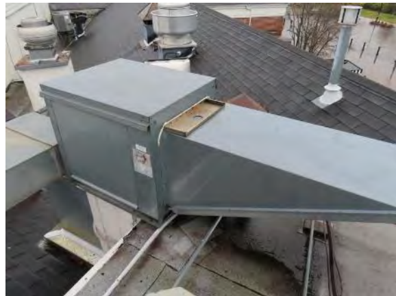
Make-up Air Unit
