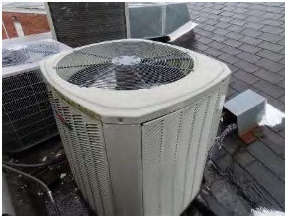
Trane 3-Ton Heat Pump Manufactured in 2014
