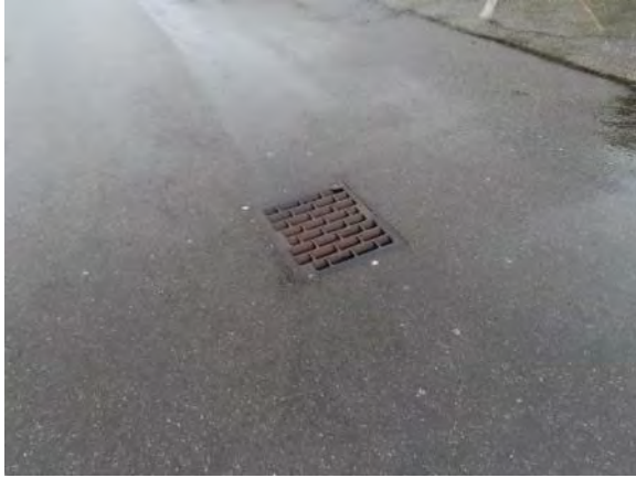
Typical Storm Drain in West Parking Lot
