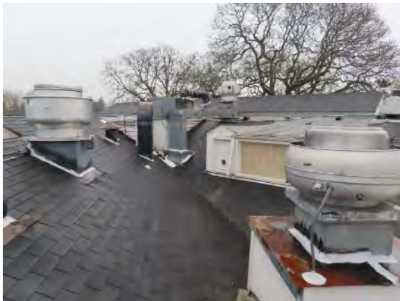
Restaurant Owned Exhaust Fans
