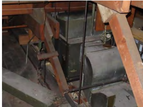
Abandoned HVAC Unit in Theater Attic
