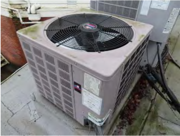
Thermal Zone 3.5-Ton HVAC Unit Manufactured in 2015
