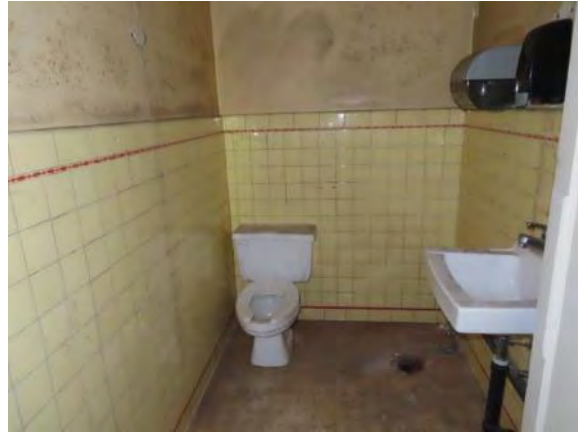
All Basement Bathrooms and Vacant Bathrooms Had Water Shut Off
