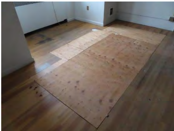
Damage to Apartment Floor
